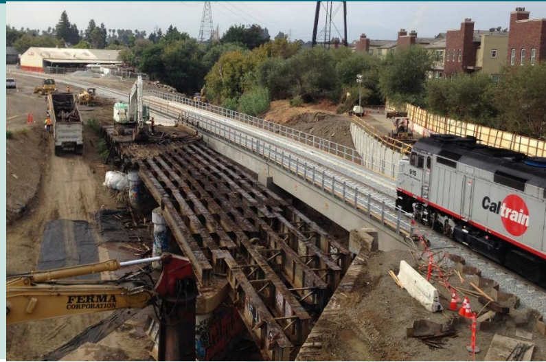
Los Gatos Creek Bridge Replacement, City of San Jose, Santa Clara County, California
